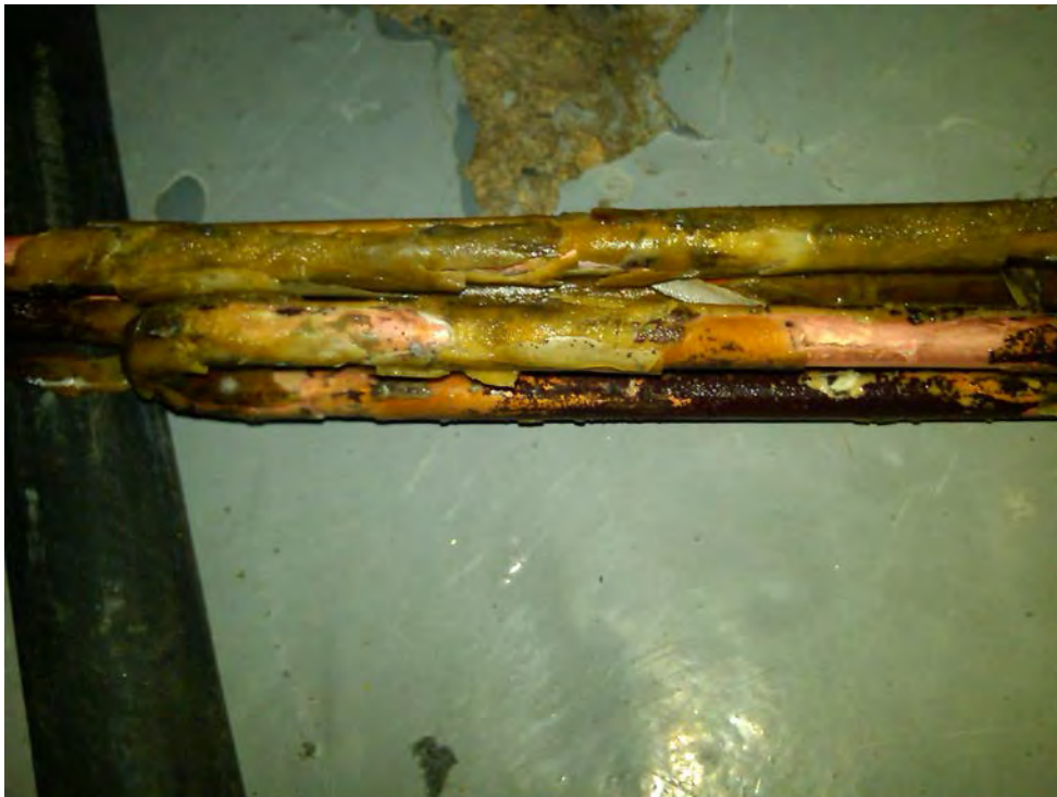
Figure 8. Heating Elements Removed June 2013.
