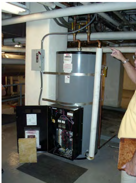
Figure 2. Electric Water Heater Where Test Was Conducted.
