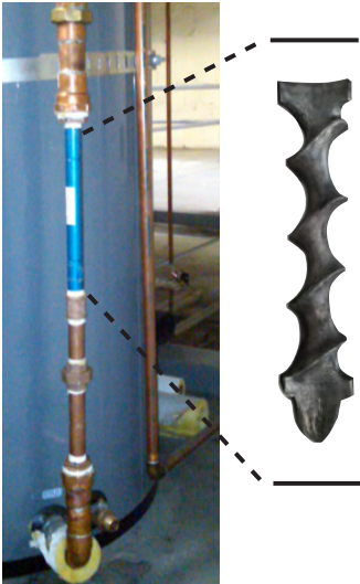
Pipe with helical insert installed in cold-water and recirculating line
